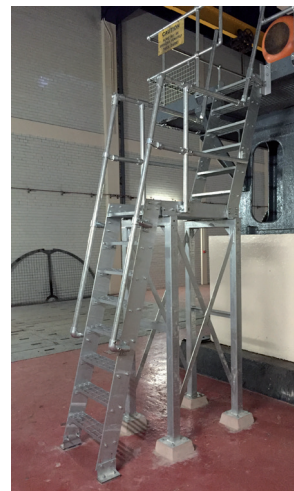
Companionway / Ships ladder over 3m with mid-height platform
