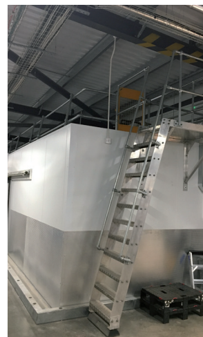
Companionway / Ships ladder with top platform
